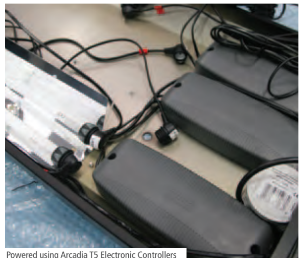
Powered using Arcadia T5 Electronic Controllers
