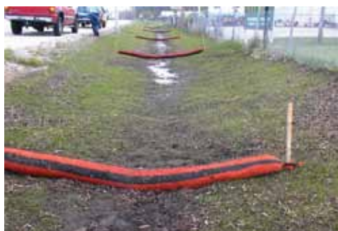
Installation of filter socks in a road ditch by Earth Corps for Indiana Department of Transportation. The filter socks will be staked through the center. Source: Filtrex International, LLC.
