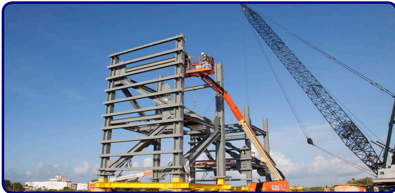
Image Caption: The first crew access tower tiers begin to take shape at Space Launch Complex-41 for flights aboard the Boeing CST-100. (Credit: NASA/Jim Grossman)
